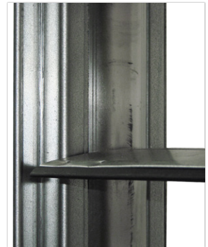
Torn aluminum jamb seals obstructing blade operation
