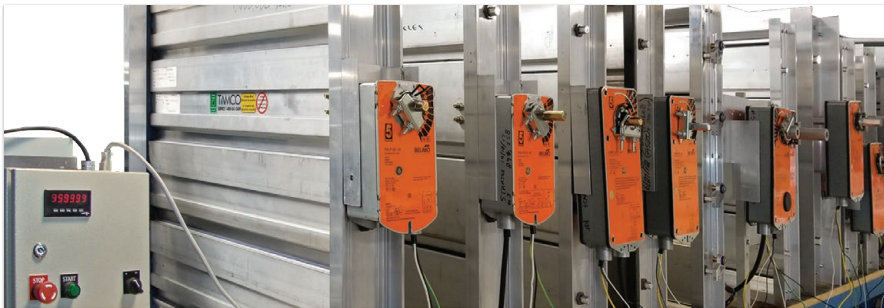
The actuators installed on each damper were connected to a timed electronic cycler.
