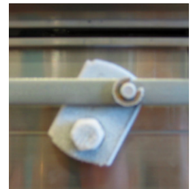
Close-up of frost build up linkage.
